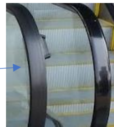
Handrail finish damage.
